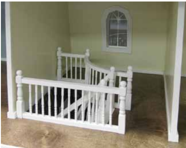
Landing Railings without trimming
